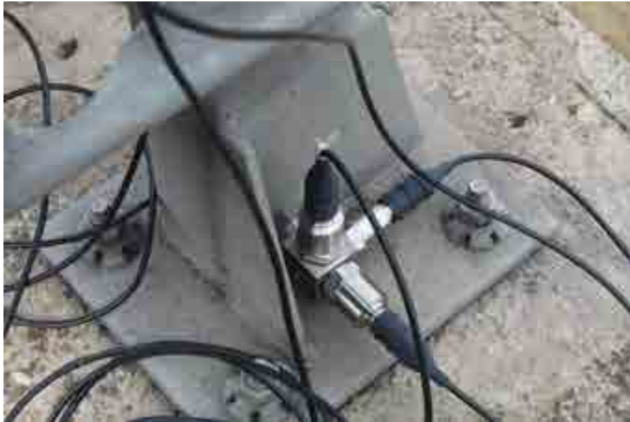
Figure 80. Accelerometer mount on the bottom part of the guardrail.
