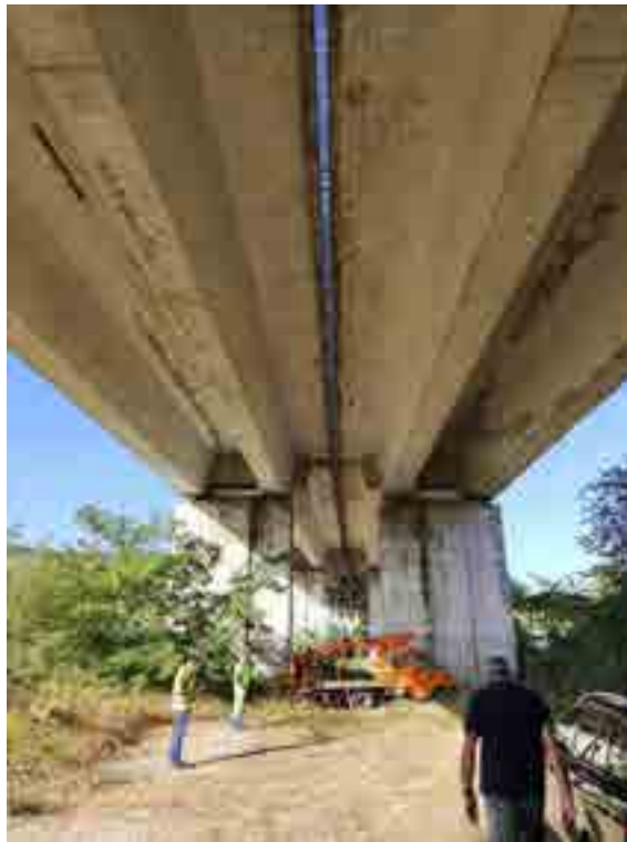
Figure 67. View from below the deck of the four box girders and the two piers that supports the second span.
