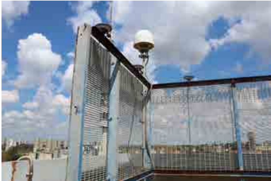
Figure 29. First view of the GNSS system configuration.
