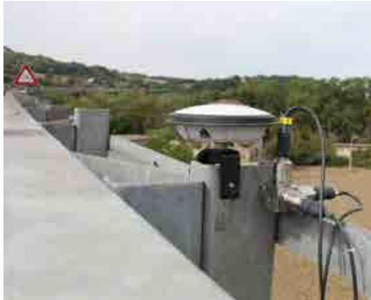
Figure 78. Antenna and accelerometer installed on the guardrail in order to monitor the same point.
