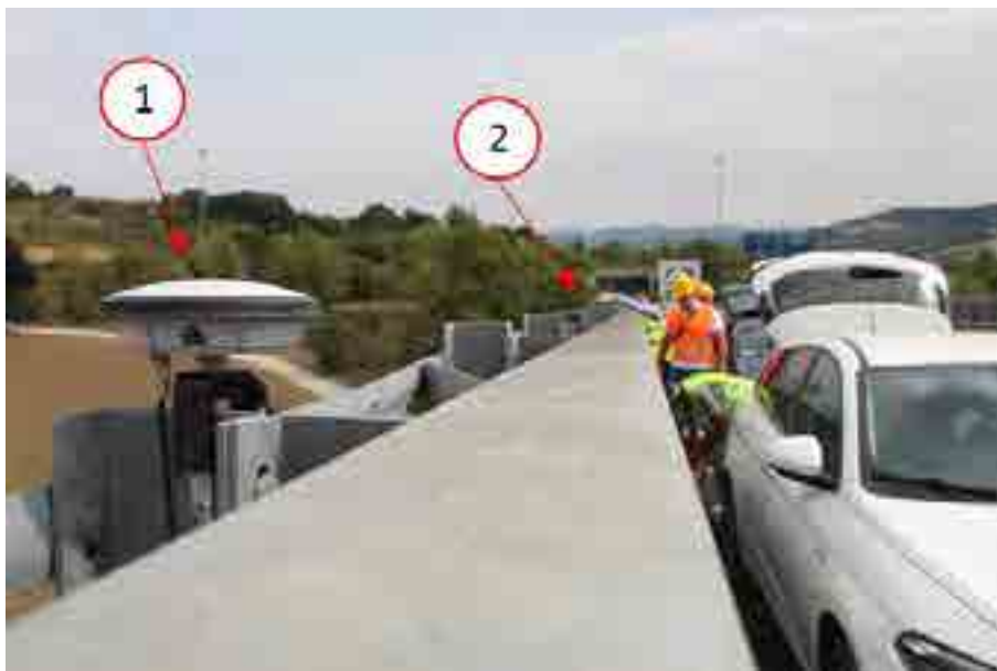
Figure 82. View of the antennas installed in the first (in foreground) and the second monitored point (in background).
