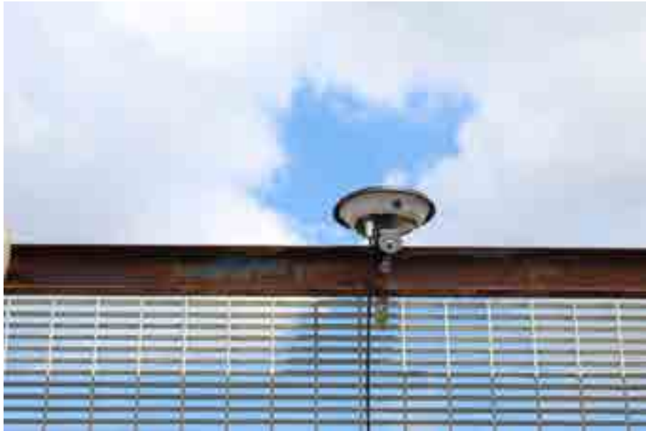
Figure 31. Third view of the GNSS system configuration.
