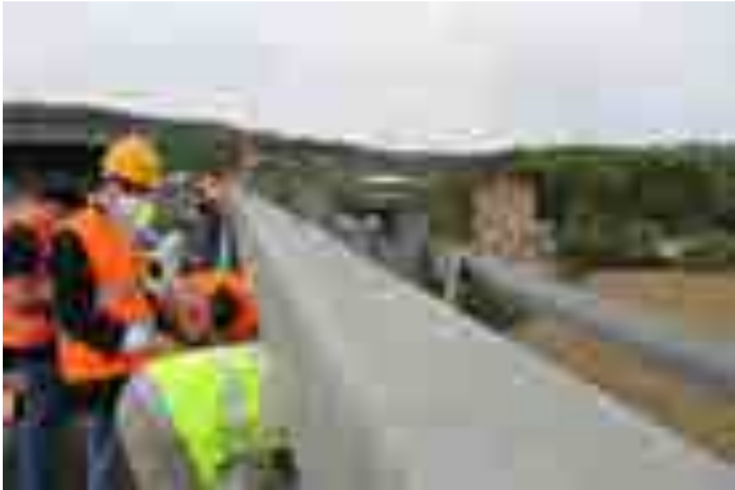
Figure 21. Installation of a GNSS antenna on the top part of the guardrail's support post.
