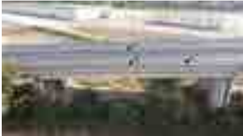
Figure 19. View of the second span of the bridge, being the monitored points highlighted.
