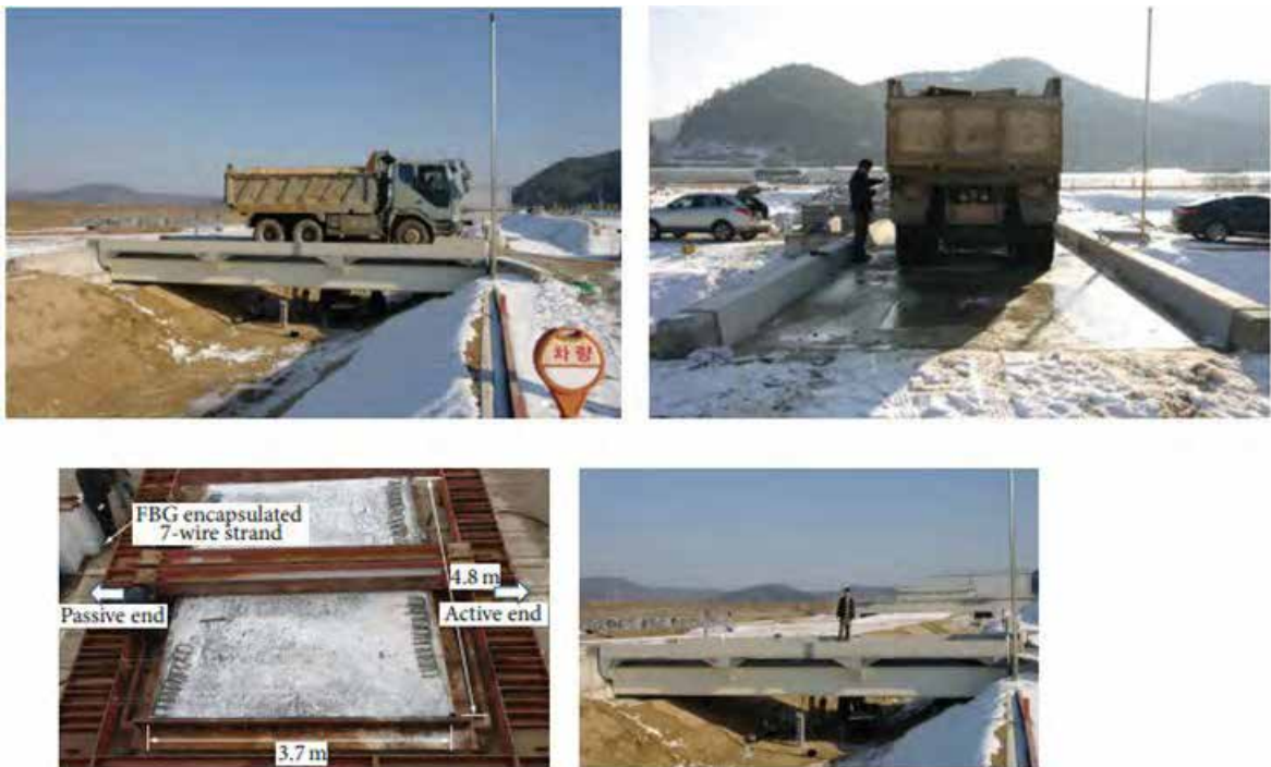
d) Bridge load test and strand internal force monitoring using FBG sensors in Korea (J.-m. Kim, Kim, Choi, & Park, 2016)
