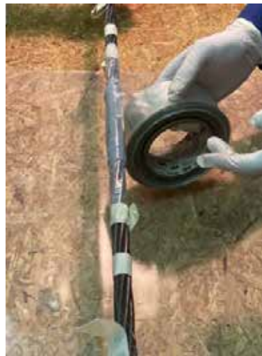
Figure 17. Covering the smart saddle with plastic sheet until to end of curing.
